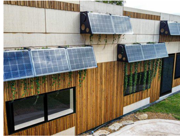
Case 2: Photovoltaic planter, Barcelona
